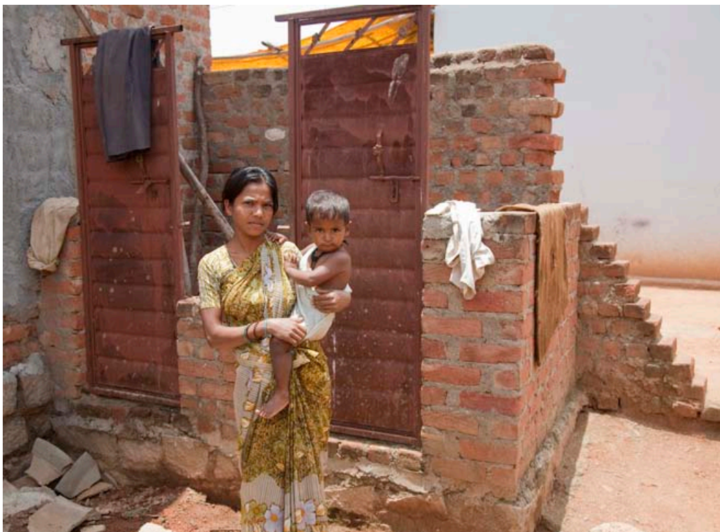
Caption: Budhari Adhavla with Bhagath outside the half built toilet and bathroom
